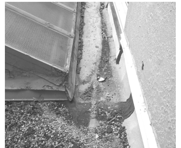
These photos show areas of weakness and places where leaking has been prevalent.
